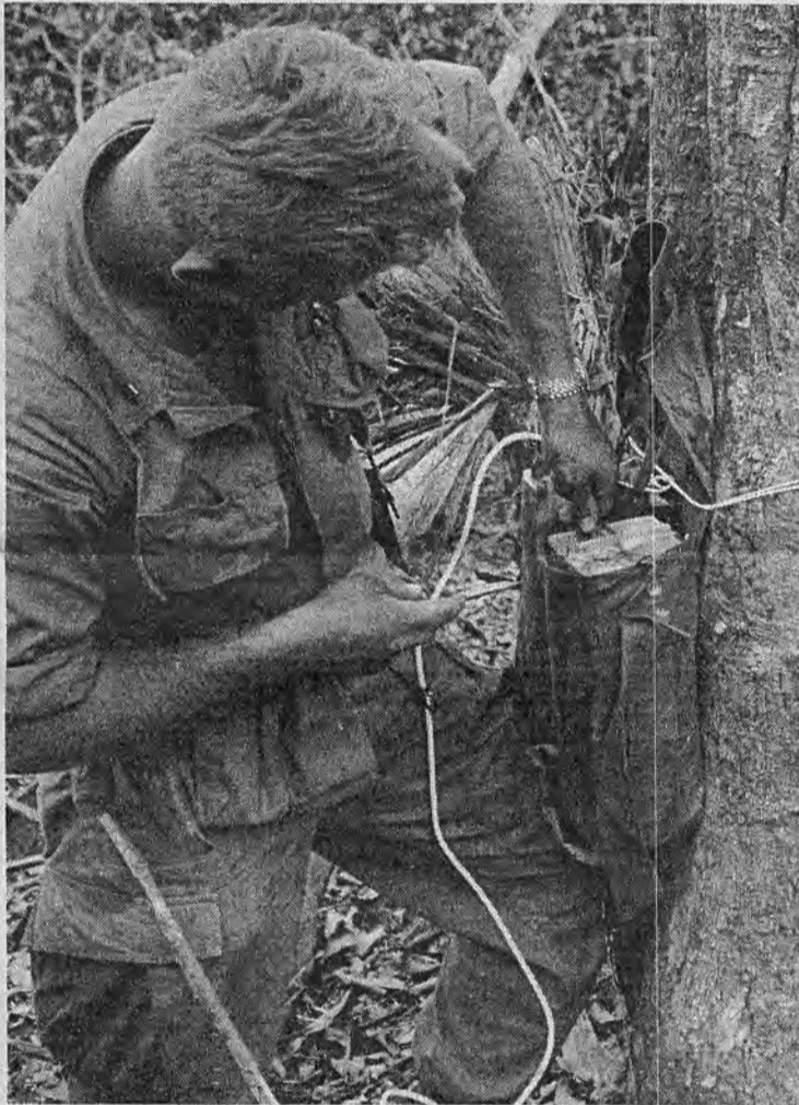
TAKING CHARGE —1LT Lynn Lysack (Des Moines, Iowa), a platoon leader with the 4th Engineer Battalion's Company A, primes a charge of plastic explosive prior to blowing another tree during the clearing of a new firebase in the jungle near Dak To. His platoon is supporting the 3rd Battalion, 12th Infantry. (USA Photo by SP4 Andy Pison)
